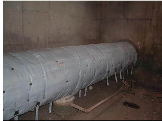
Double Slip Expansion joint & Piping
