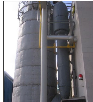
Gas Turbine Exhaust Silencer
